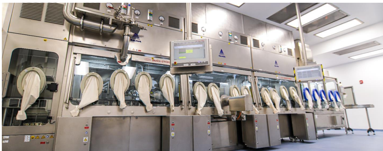
Figure 2: VarioSys® Aseptic Fill Line
